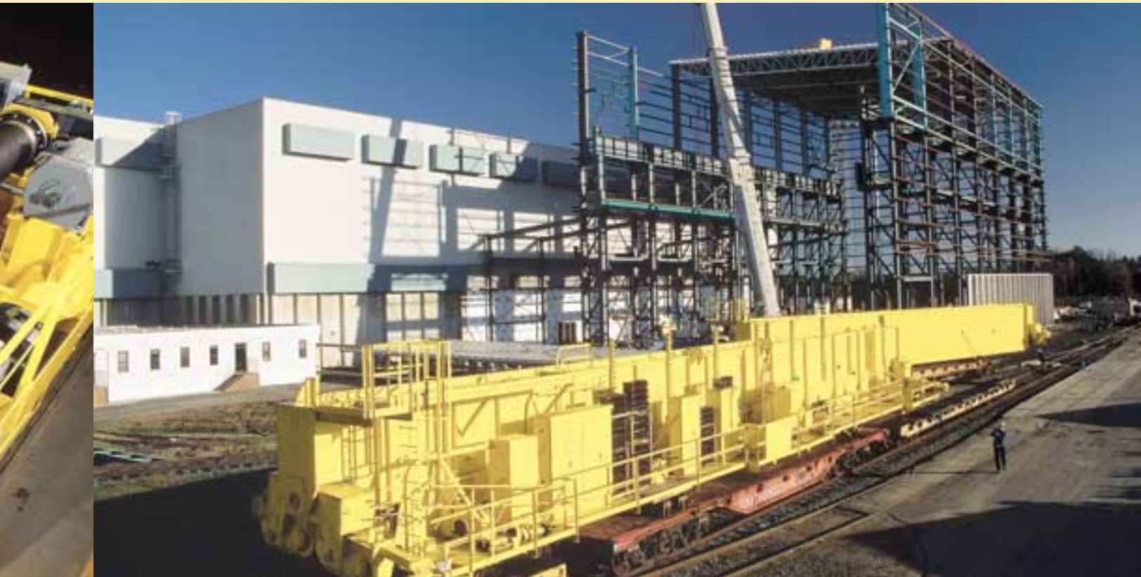
A 700-ton bridge crane owned by Siemens Westinghouse Power Inc. was renovated by Konecranes Engineered Services, and then relocated from Tampa to The Siemens Westinghouse Turbine Generator Plant in Charlotte by rail.
