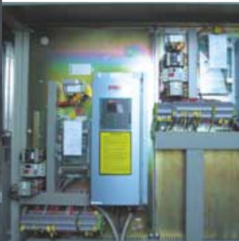
Modern AC inverter system, DynAC and DynAHoist.
